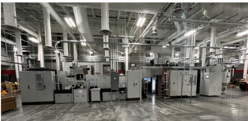
Pictured is new Inspection Finishing System (IFS) Equipment installed at the Western Currency Facility. The IFS uses sophisticated sensor and camera systems to reclaim unfit currency notes from currency sheets produced in the previous printing operation.
